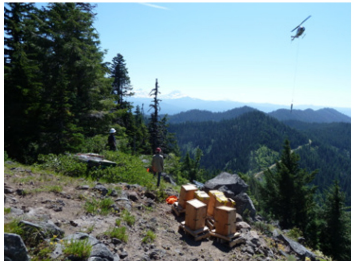
A helicopter delivers supplies for the construction of a WiFi tower at the top of Roswell Mountain at the Andrews Forest. The tower will be part of a wireless connection across much of the Andrews Forest site. Photo by Jay Sexton.
