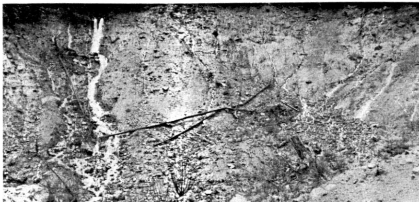
AFTER PROLONGED RAINS, water literally squirts out of road cuts from top to bottom.
