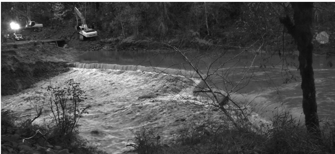
Figure 2. Knickpoint migration after cofferdam notch. The lateral (river right) and longitudinal (river left) arcuate knickpoints have migrated several meters from the cofferdam notch (located just out of the picture on the left). photo credit: J. Rose Wallick
